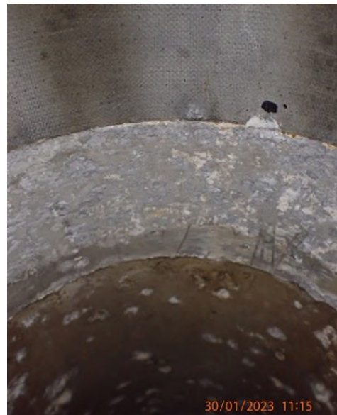
Figure 17 – Port Fwd Location 1 (12 O'clock) Corrosion 6M
