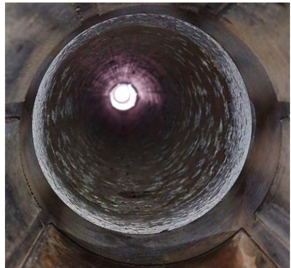
Figure 15 – Port Fwd Sleeve 6M Corrosion (High Pressure Washed)
