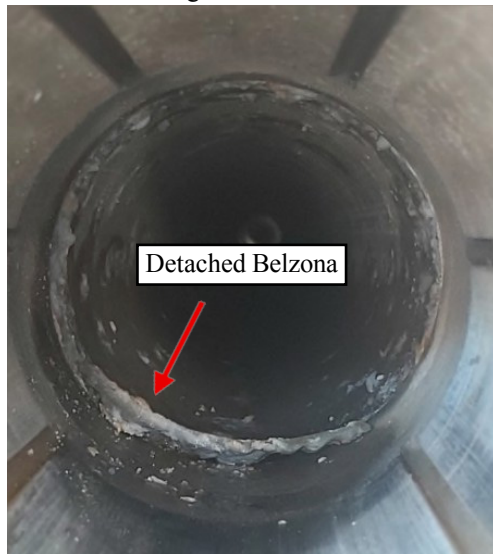
Figure 6 – Mid Port bearing inspection with detached Belzona section blocking cooling water flow (6 o'clock)
