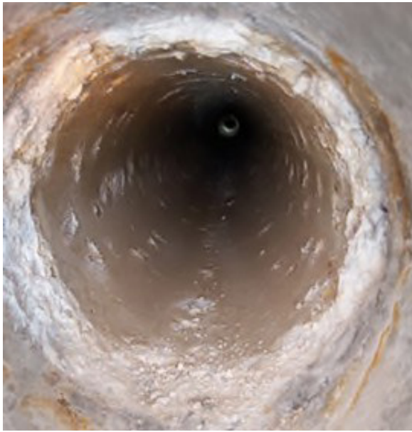
Figure 3 – Stern tube corrosion around bearing housing recess interface
