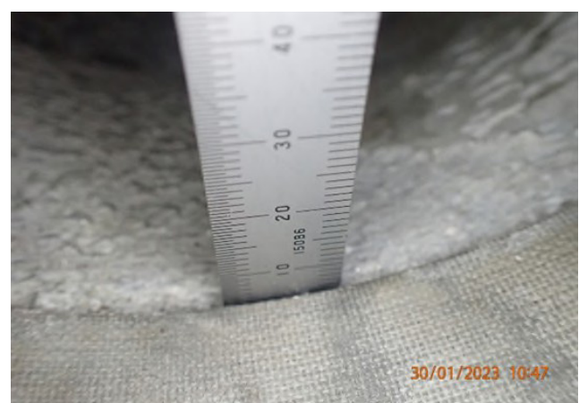
Figure 25 – Stbd Fwd Location 3 (6 O'clock) Corrosion 6M
