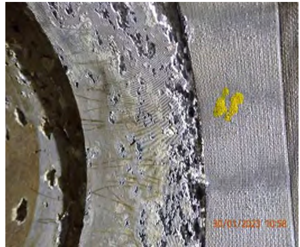
Figure 21 – Stbd Fwd Location 1 (12 O'clock) Corrosion 6M
