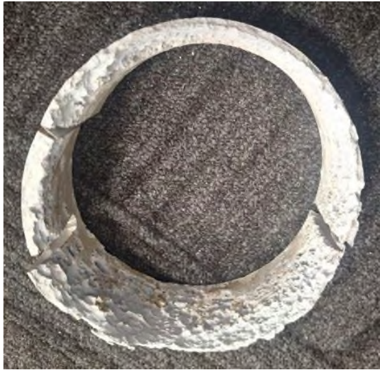
Figure 26 – Sacrificial sleeve mating face with bearing recess 22M corrosion
