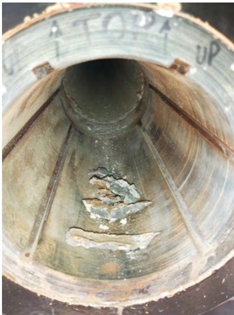
Figure 8 – Stern tube with detached Belzona debris
