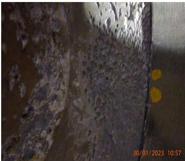
Figure 22 – Stbd Fwd Location 2 (3 O'clock) Corrosion 6M
