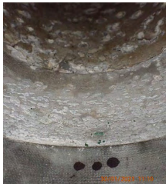
Figure 19 – Port Fwd Location 3 (6 O'clock) Corrosion 6M
