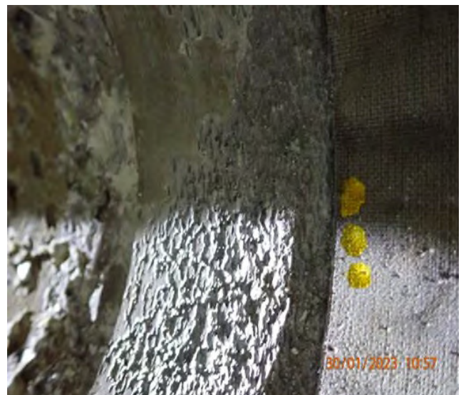
Figure 23 – Stbd Fwd Location 3 (6 O'clock) Corrosion 6M
