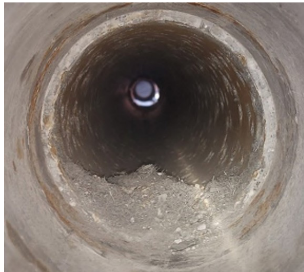
Figure 29 – Sacrificial sleeve external condition 22M
