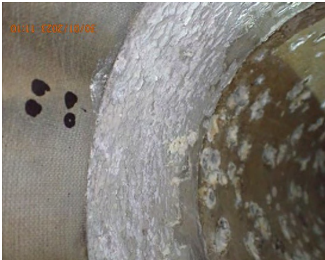
Figure 20 – Port Fwd Location 4 (9 O'clock) Corrosion 6M
