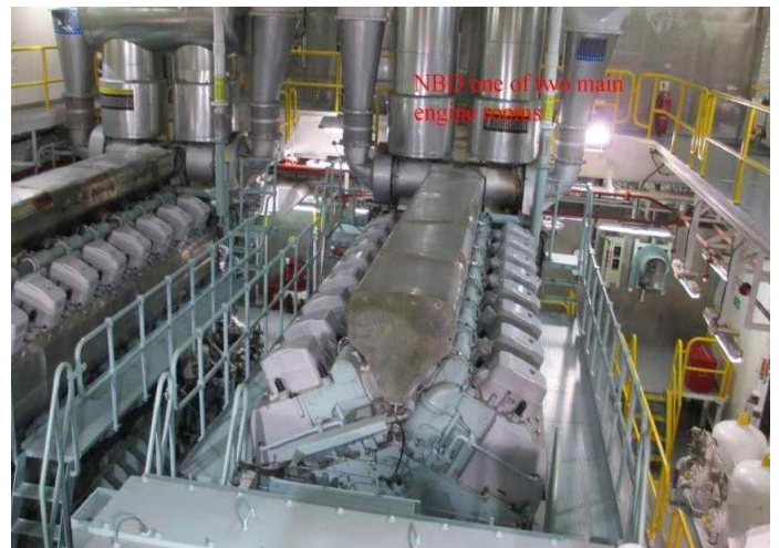
NBD one of two main engine rooms
