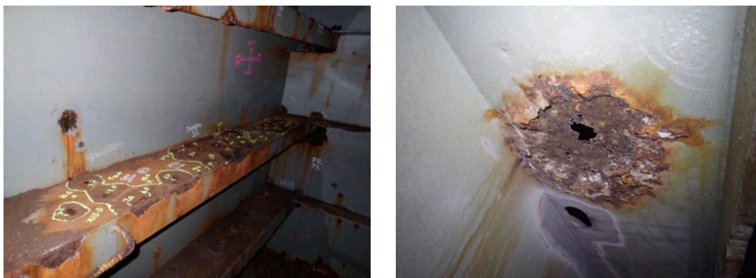
Figure 2 Anomalies as found during the original tank inspection and prior to repair
